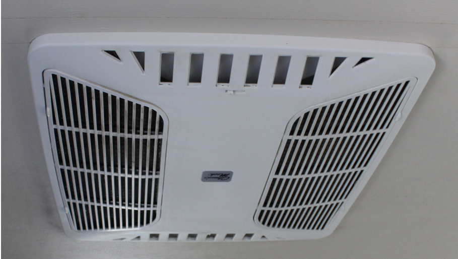
AC overhead vent
