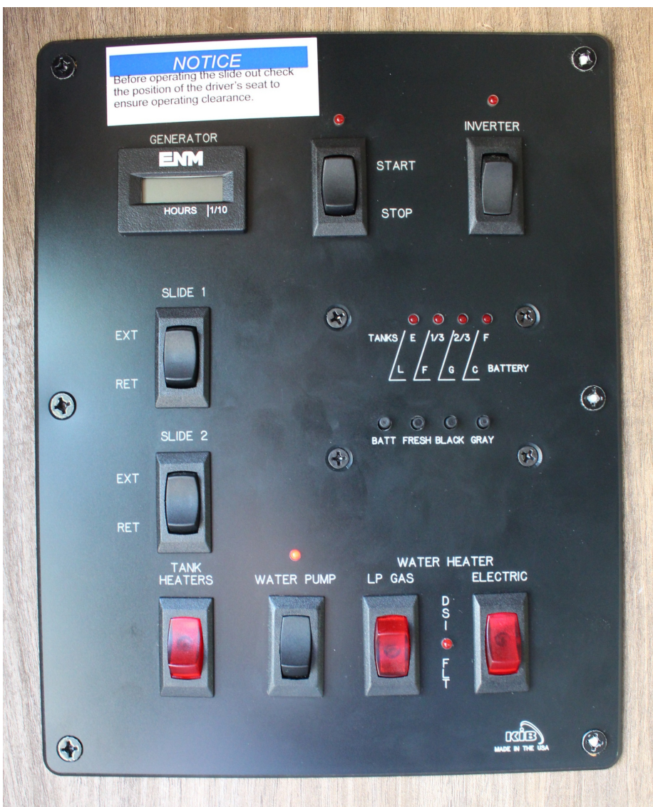
Main Control Panel: slides generator water heater tank guage tank heater
